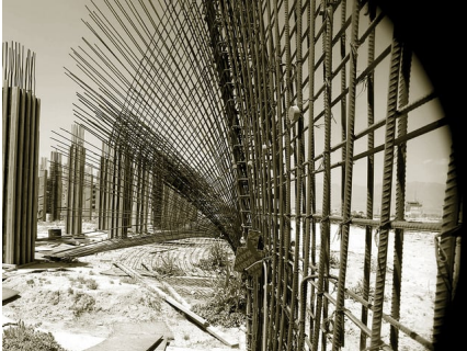
Tilted columns and sagging reinforcing rods at the Justice Center Court House construction project in Parwan Province, Afghanistan. (SIGAR via Flickr )
